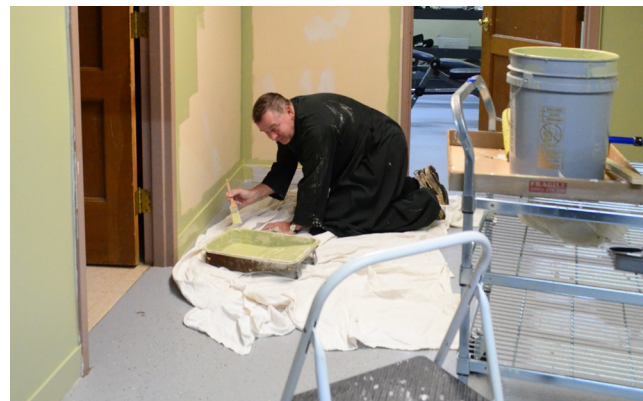
Brother Peter Joseph applies a new coat of paint to the walls of the Novitiate basement.
